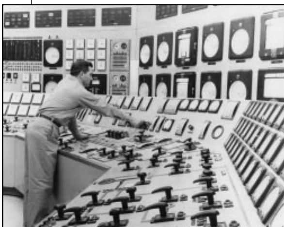
Nuclear reactor control room.
